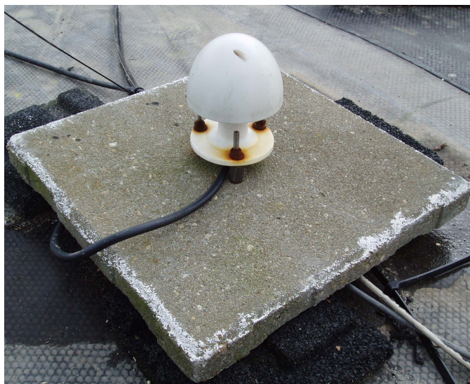
Figure 2.2: The GPS antenna is mounted on the plastic anchor. To prevent modifications to the roof, the anchor is secured by a weight (tile).
